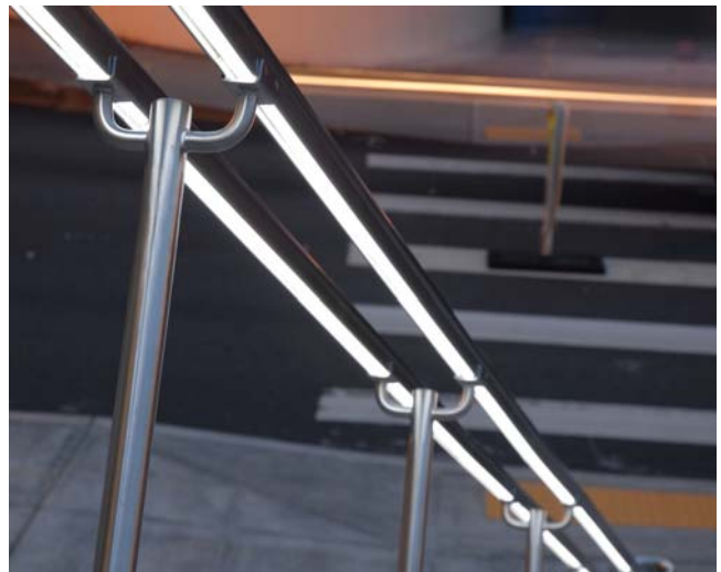
Designers: Mazzetti Nash Lipsey Burch (M+NLB), Perkins & Will, and Petersen, Kolberg & Associates Photograph: Hanset Corporation
